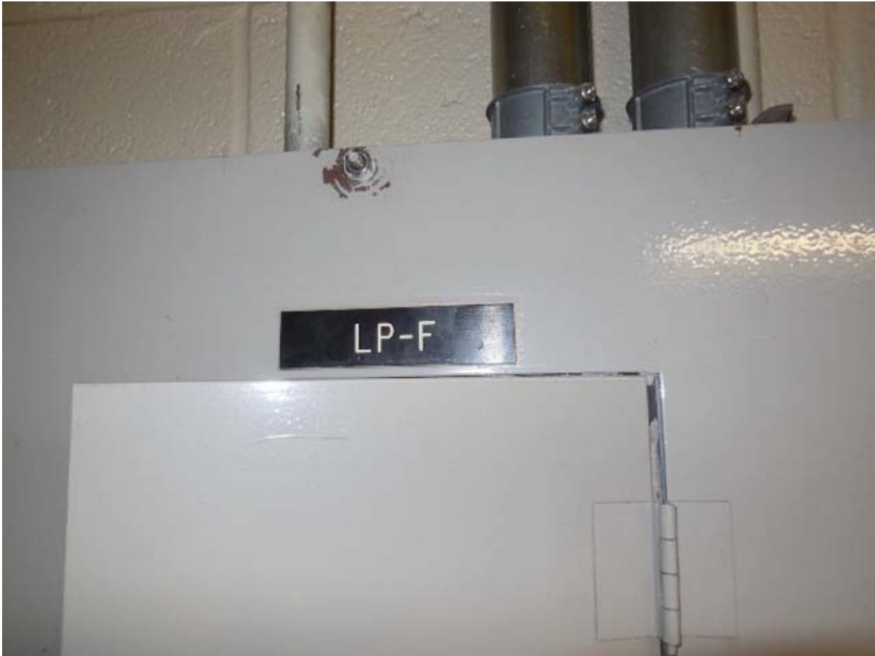
Picture 9: D13 New Carrollton – Panel LP-F in Room C106
