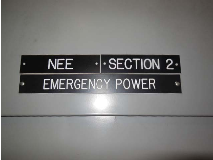
Photo #8: J02 Van Dorn Street – Label for Kiosk Emergency feed Source Panel NEE in Room 110
