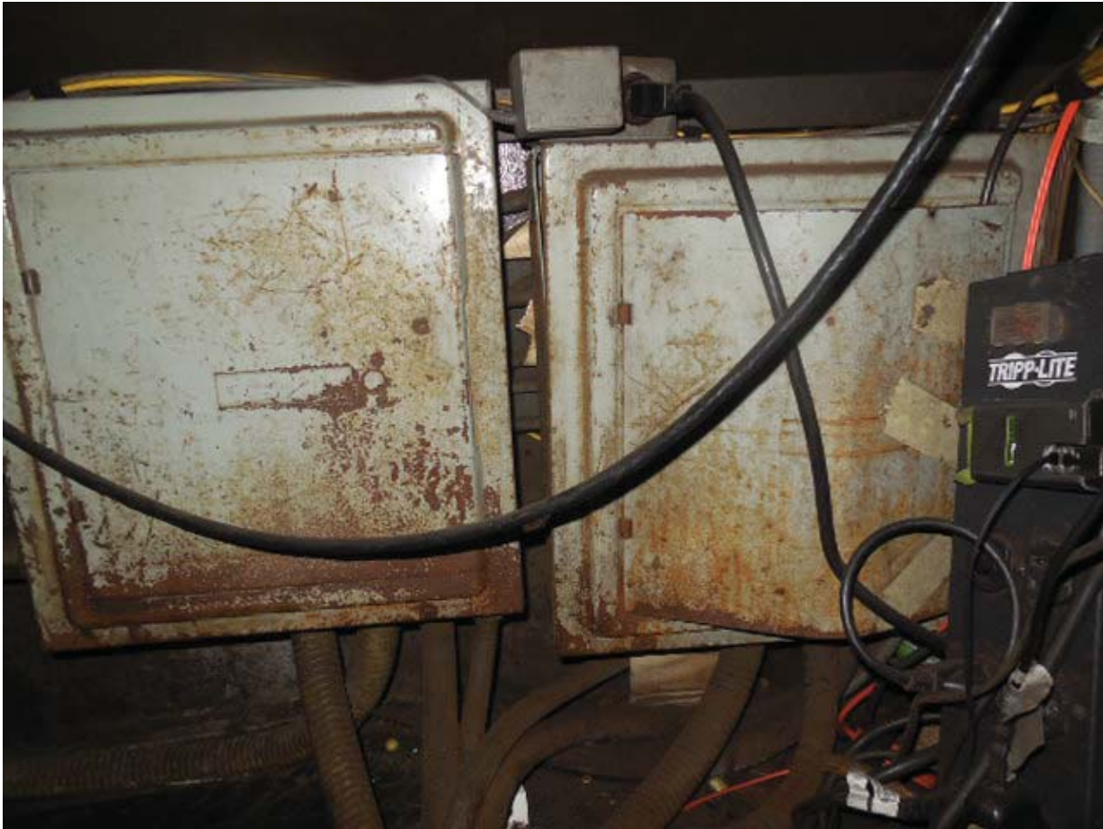
Picture 3: G01 Benning Road – Emergency panels in Kiosk
