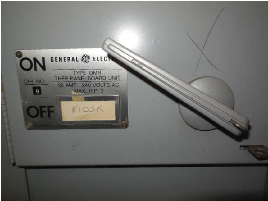
Photo #9: J02 Van Dorn Street – Label for Kiosk Emergency feed Source Breaker “Kiosk” in Room 110
