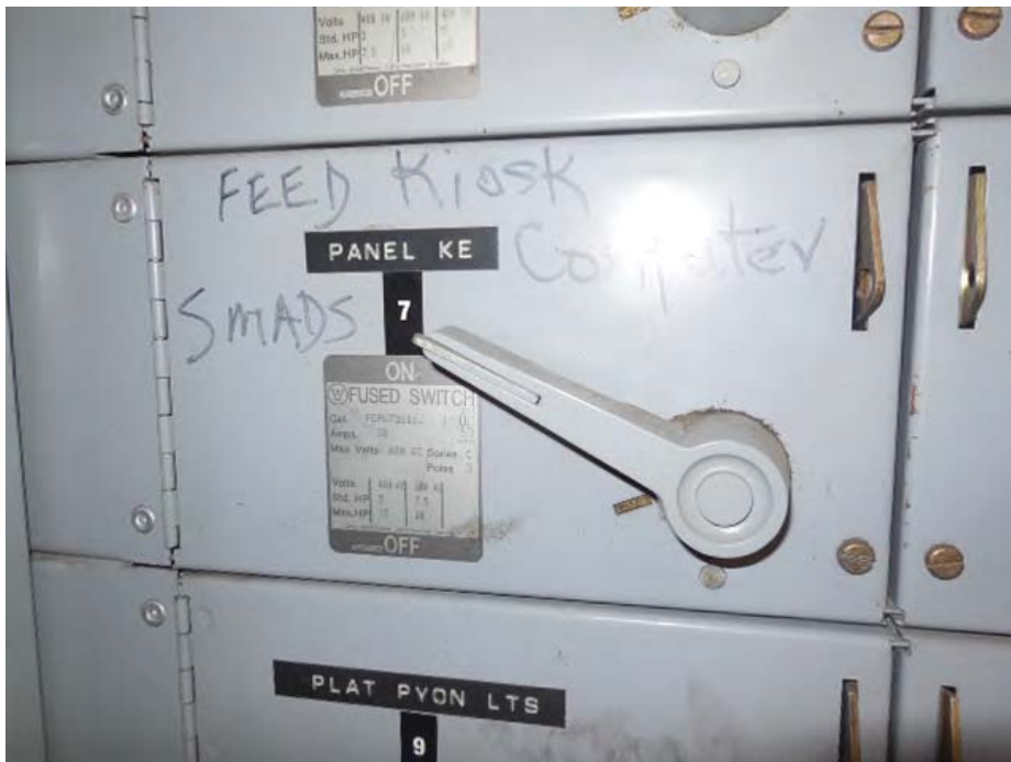
Photo #12: J03 Franconia-Springfield – Emergency feed for Kiosk Panel – Circuit Switch for Panel KE
