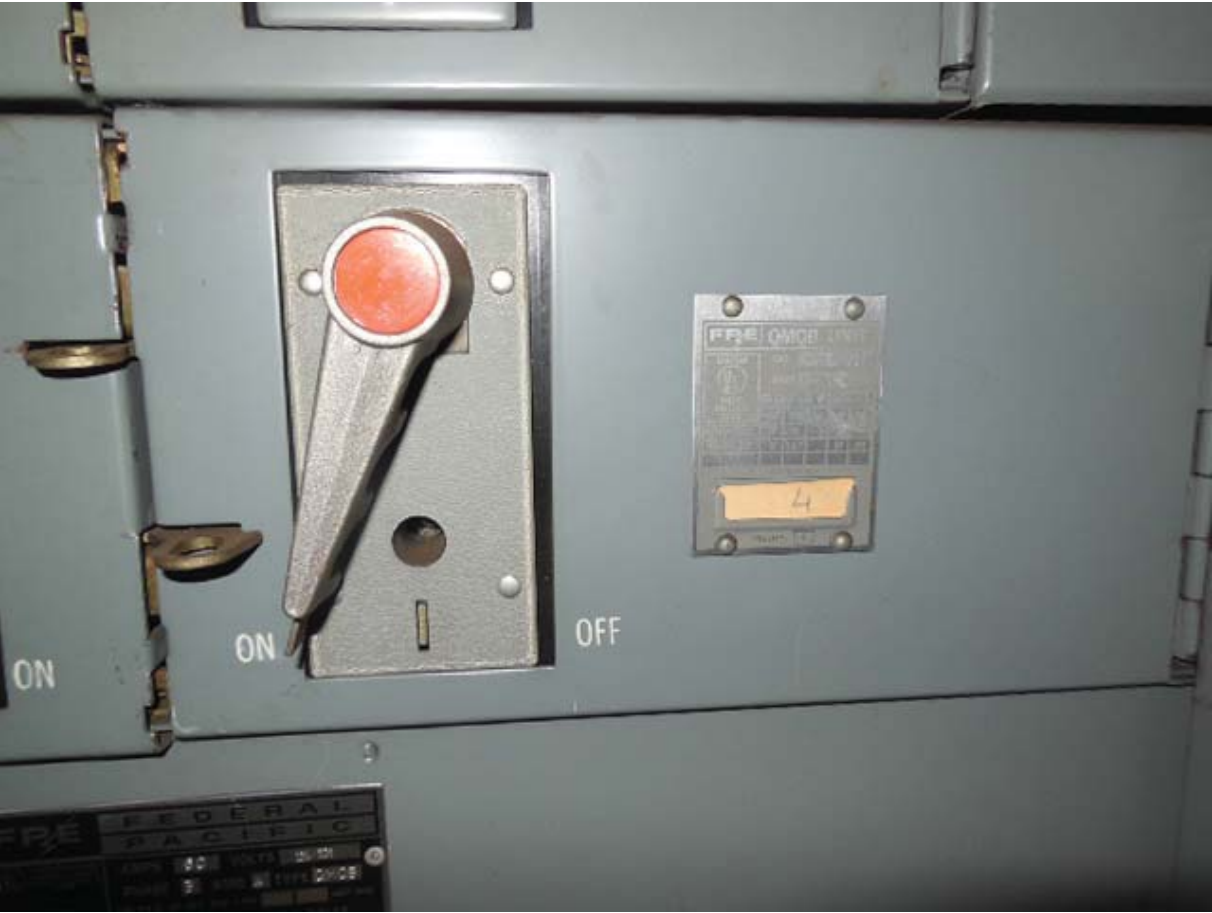
Picture 12: G03 Addison Road – EP02B Emergency Power Panel in Room 207 – Circuit 4
