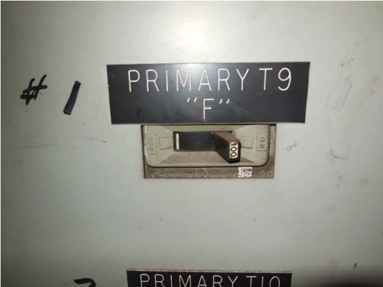
Picture 10: G03 Addison Road – Primary T9 “F” Disconnect Switch in Room 207
