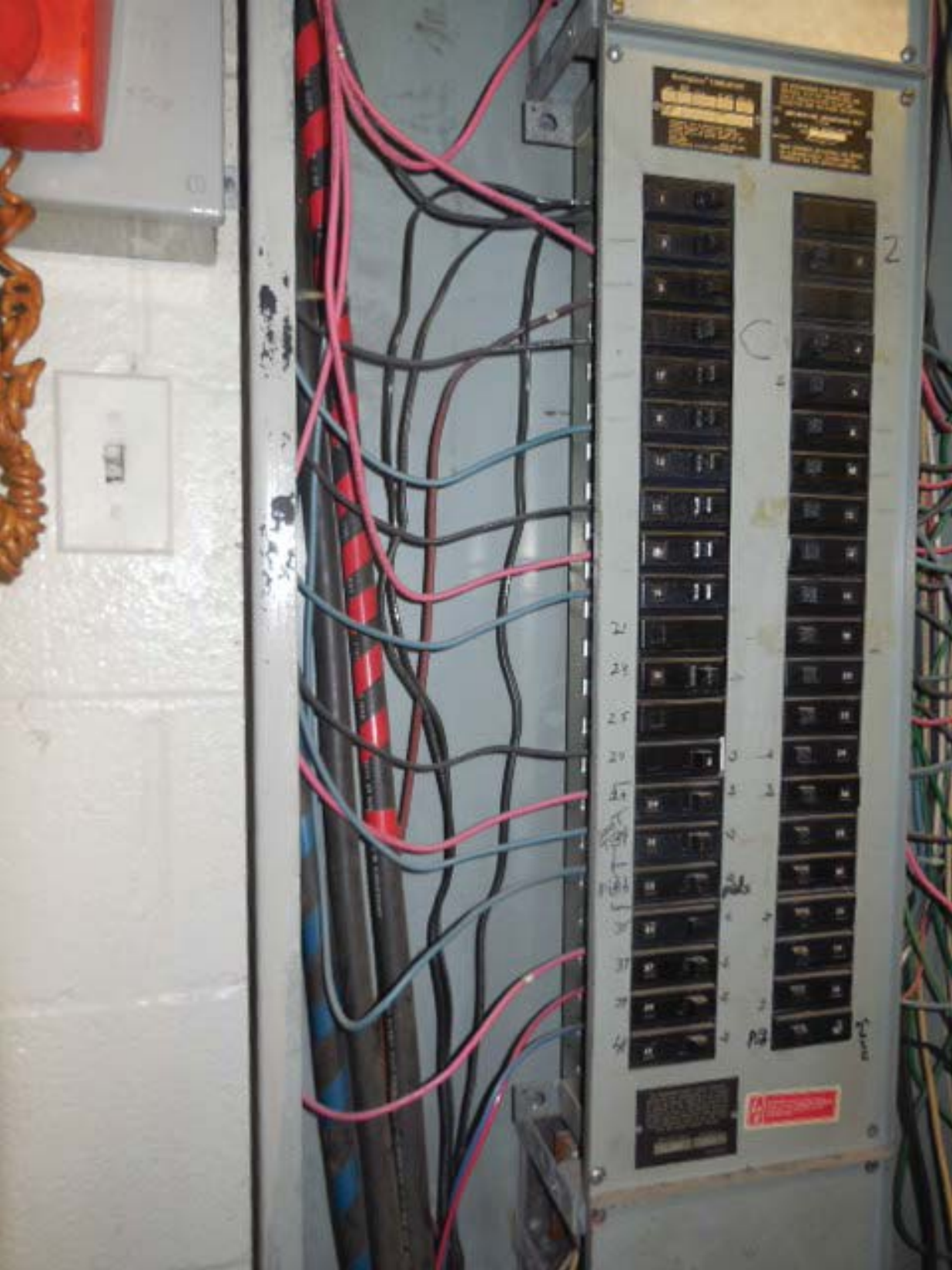
Picture 10: D13 New Carrollton – Panel LP-F in Room C106
