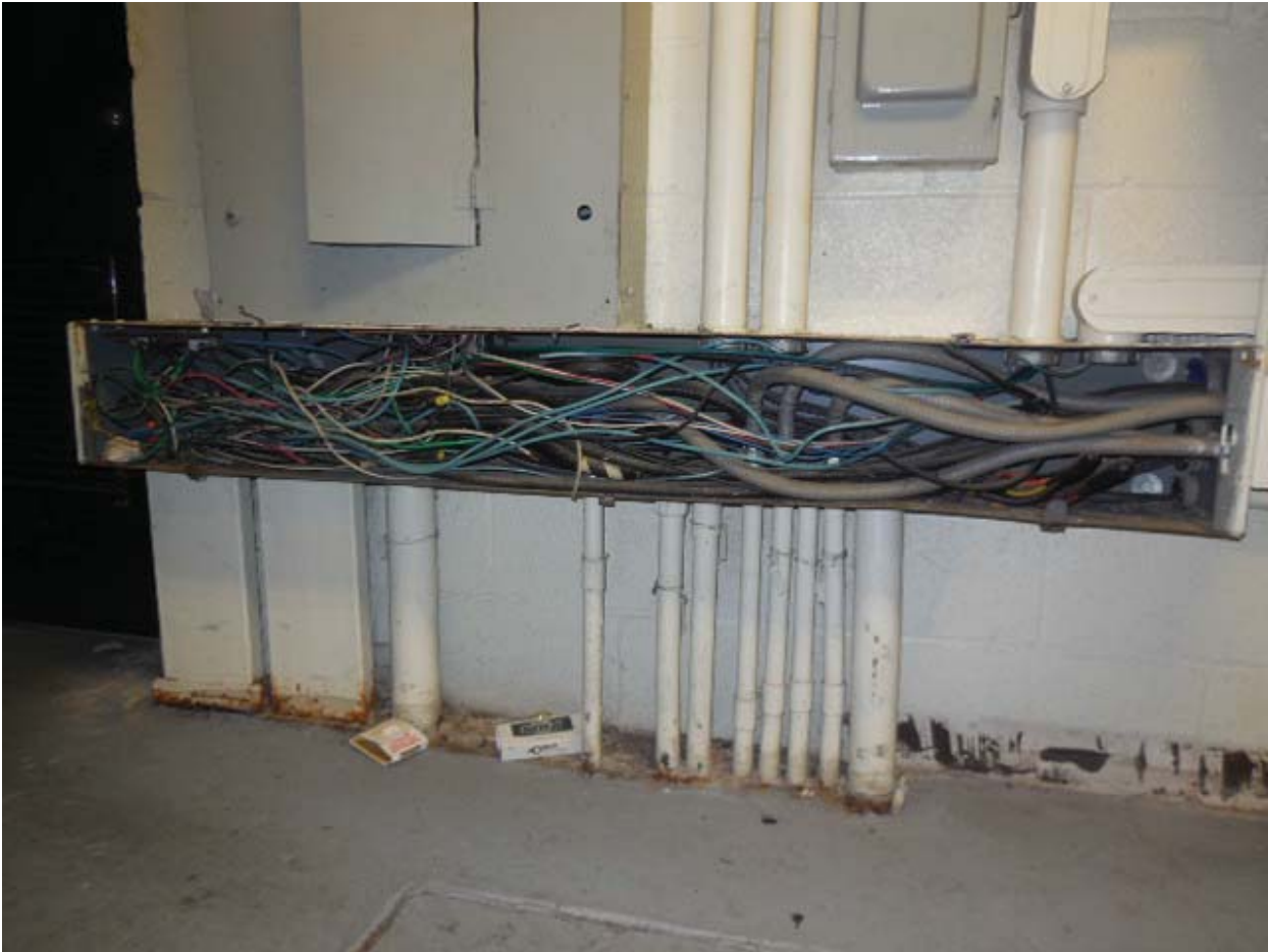
Picture 8: D13 New Carrollton – Common trough for Panels LP-F, LP-E and LP-EM in Room C106
