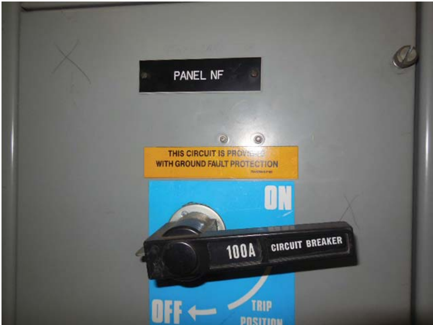
Photo #7: J02 Van Dorn Street – Source breaker for AFC panel NF in Room 110
