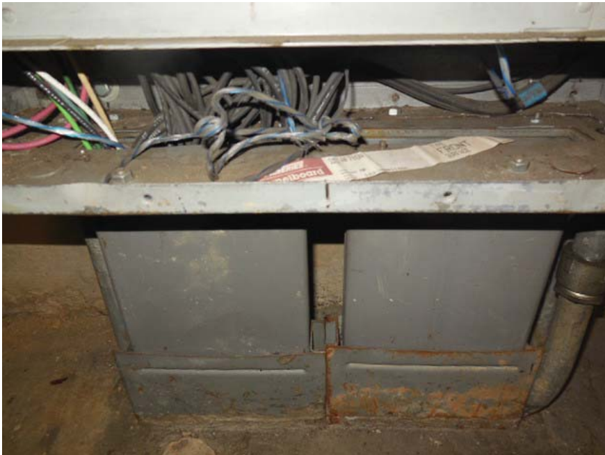
Photo #4: J02 Van Dorn Street – Bottom of AFC panel NF in Room 110
