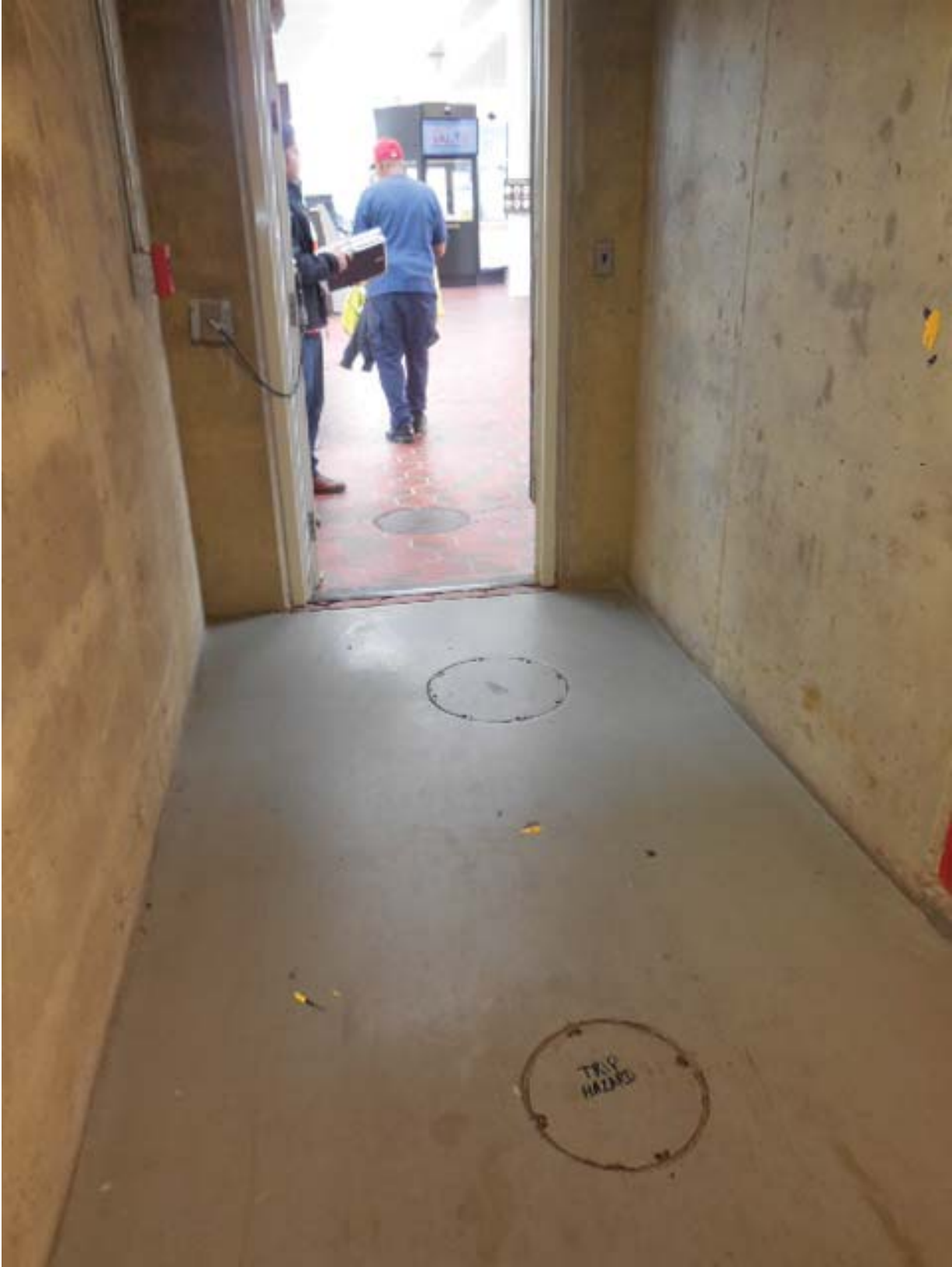
Picture 3: G04 Morgan Boulevard – Manholes in Mezzanine
