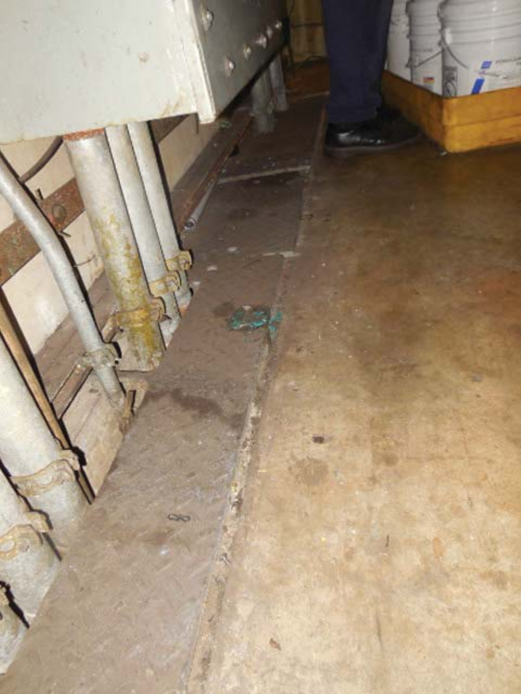
Picture 19: G02 Capitol Heights – Common trench in room 206
