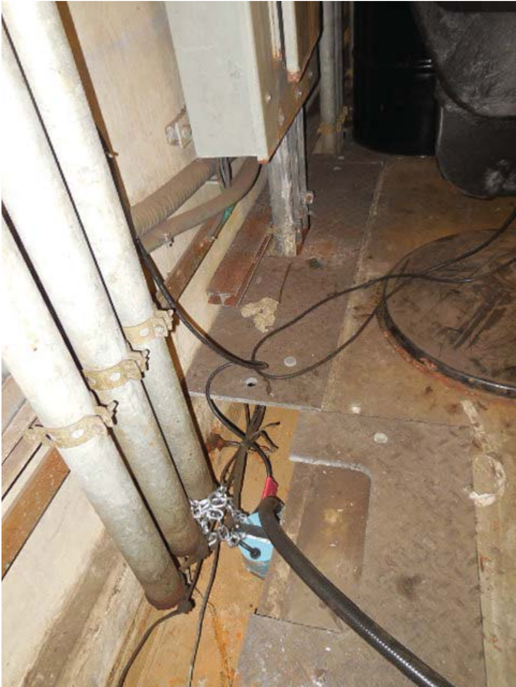
Picture 18: G02 Capitol Heights – Common trench in room 206
