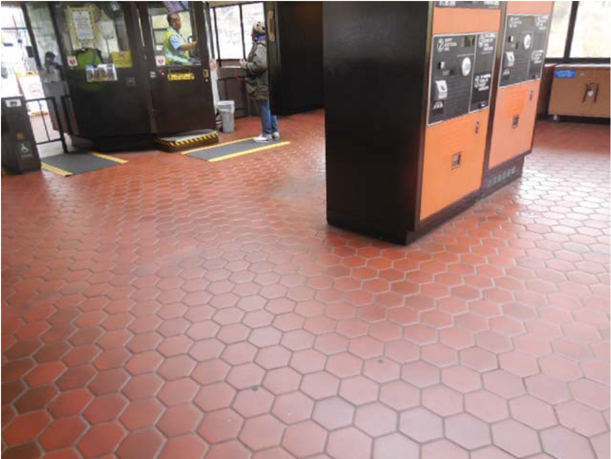
Picture 2: G03 Addison Road – No handholes in Mezzanine
