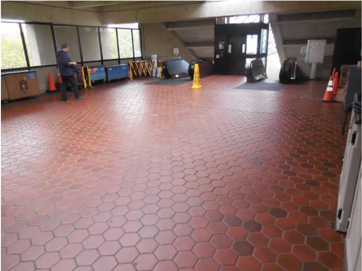
Picture 1: G03 Addison Road – No handholes in Mezzanine
