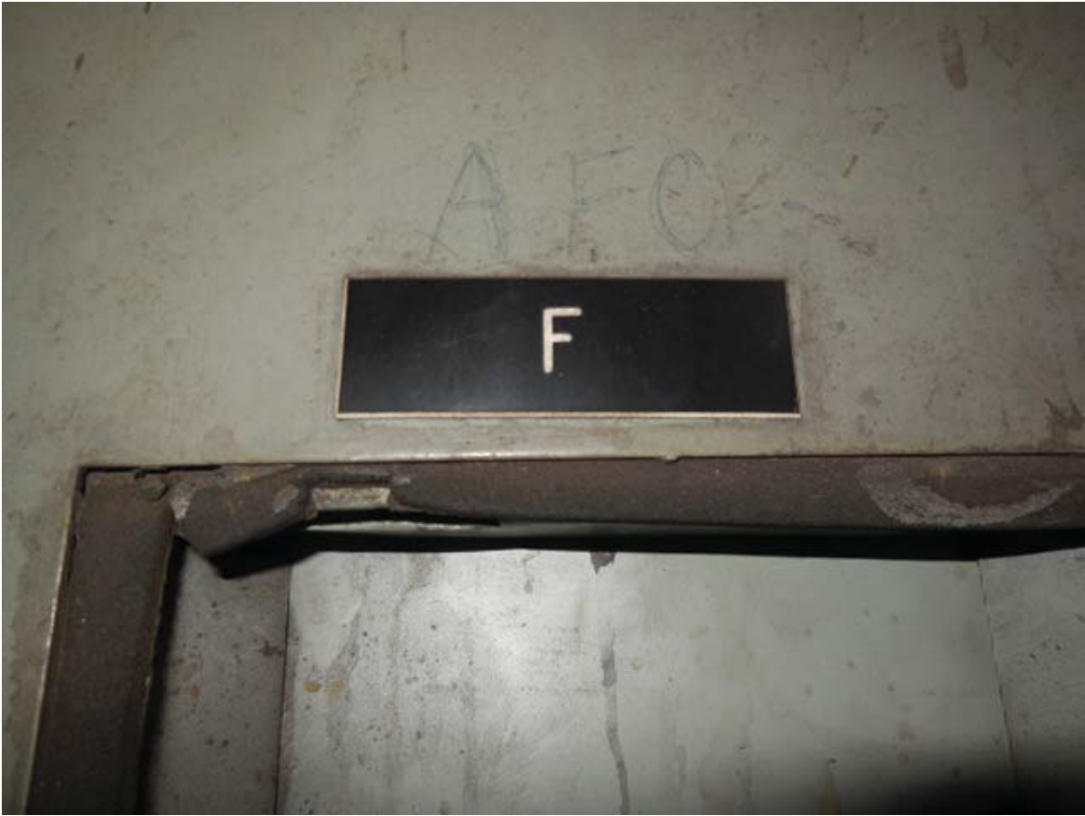
Picture 6: G01 Benning Road – AFC Panel F in Room 102
