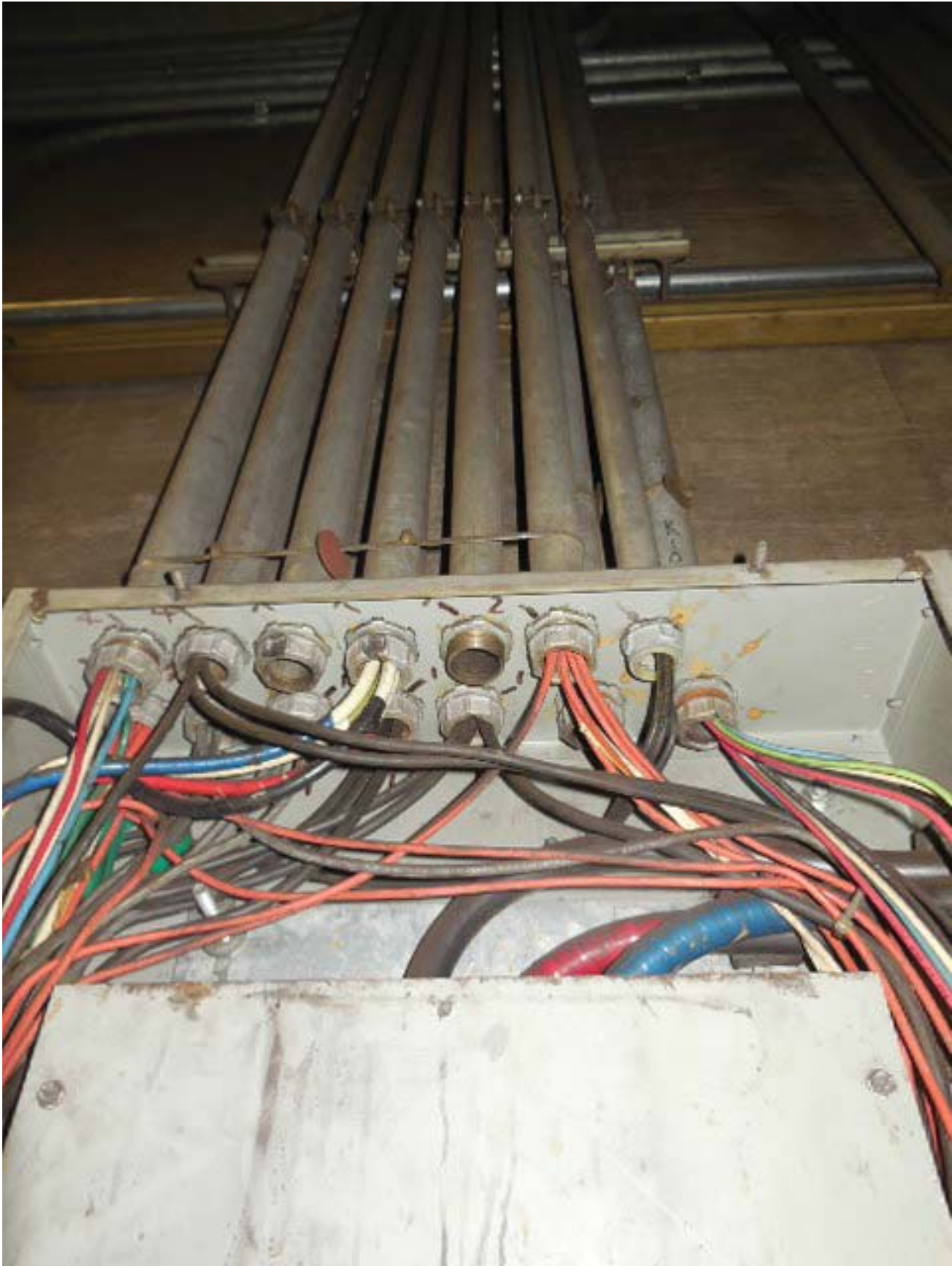
Picture 10: G01 Benning Road – AFC Panel F in Room 102 – Conduits above panel
