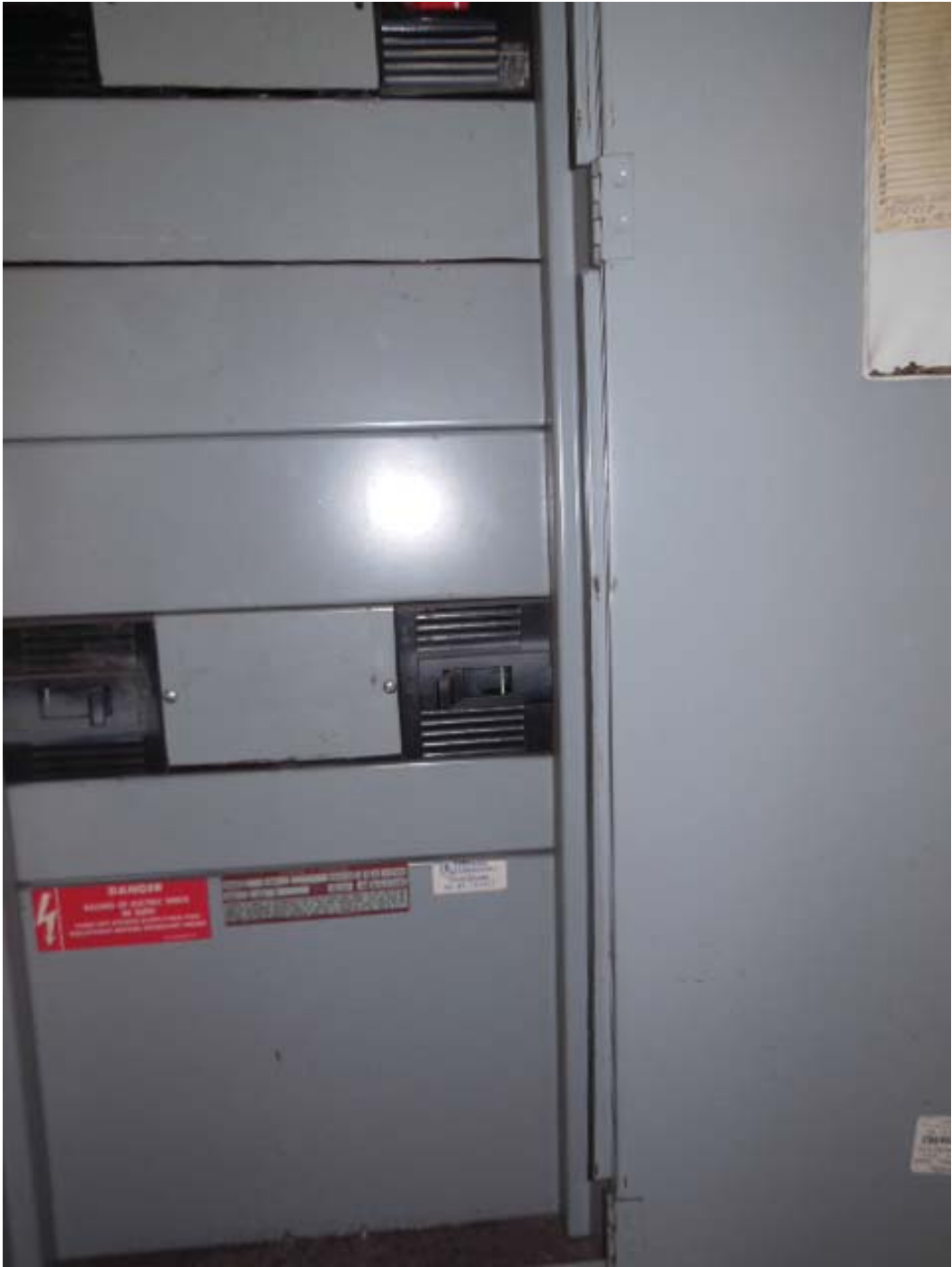
Picture 15: G02 Capitol Heights – Panel MPOE in room 206 – Circuit #4
