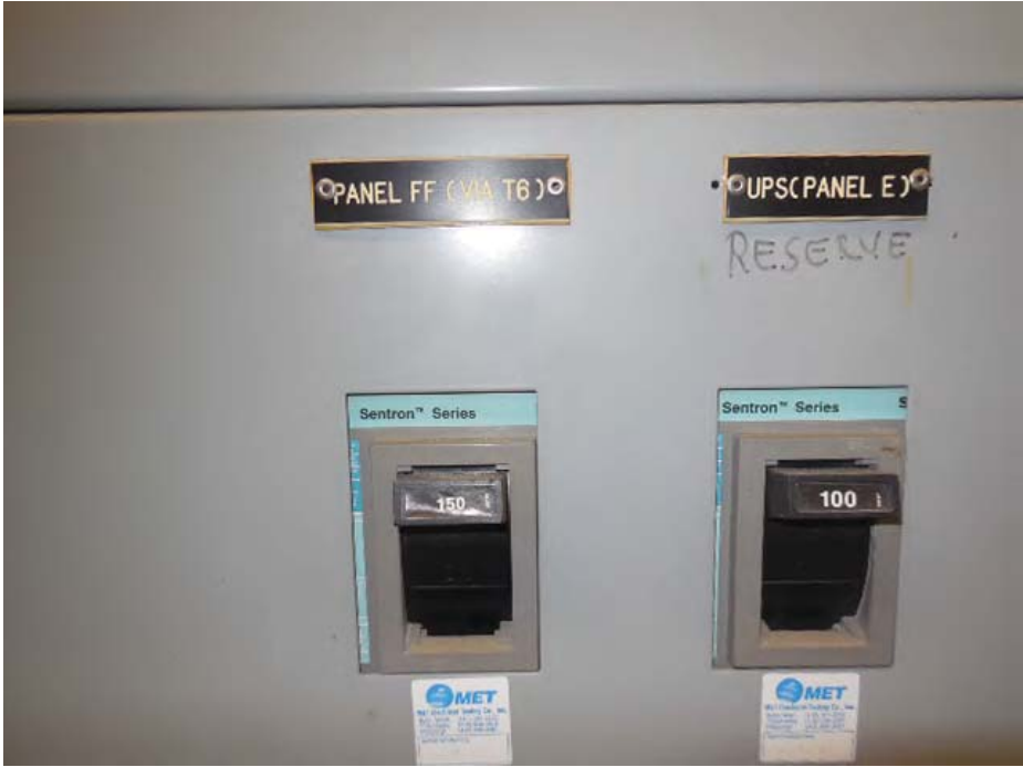
Photo #10: J03 Franconia-Springfield – AFC Panel circuit on Switchboard #2 in room 216
