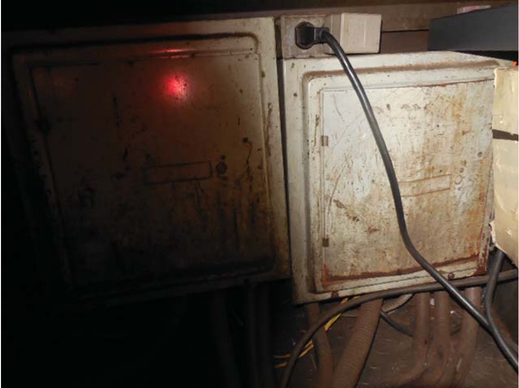
Picture 3: G02 Capitol Heights – Emergency panels in Kiosk
