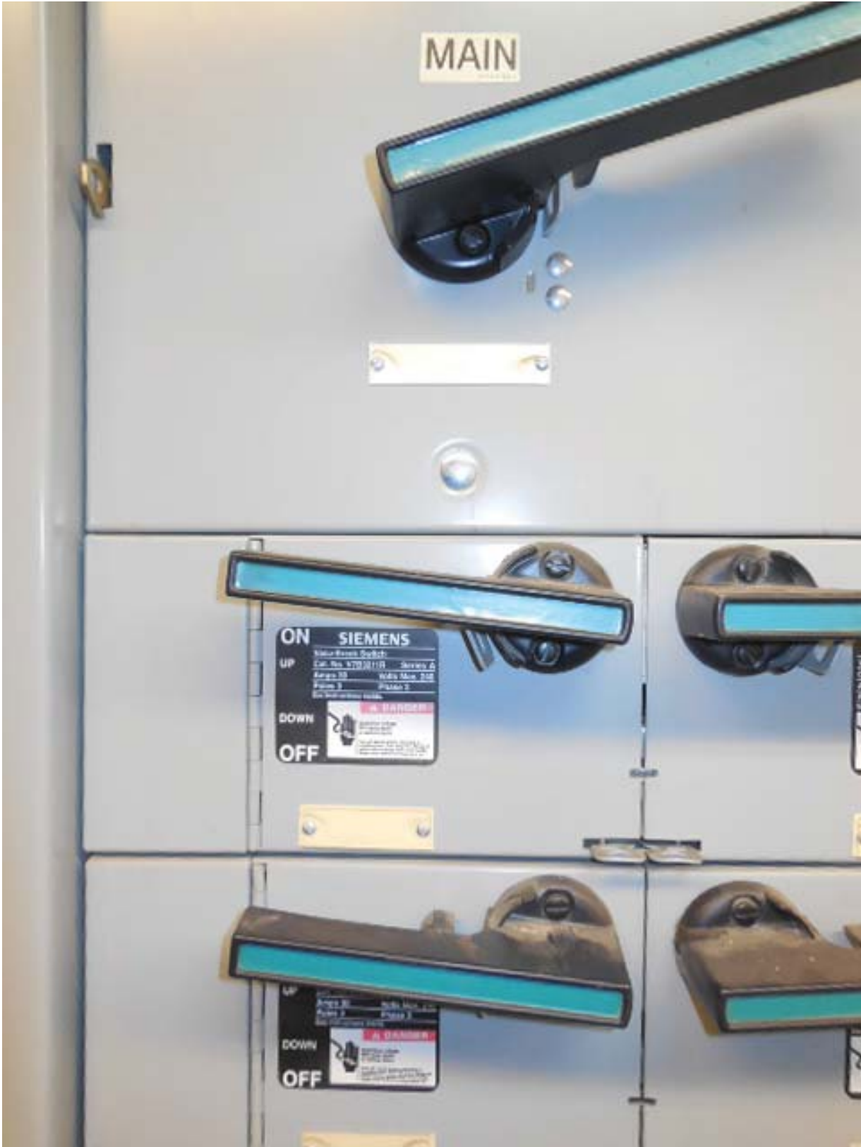
Picture 12: G04 Morgan Boulevard – Emergency Panel WMEE in Room 205 – Circuit 3
