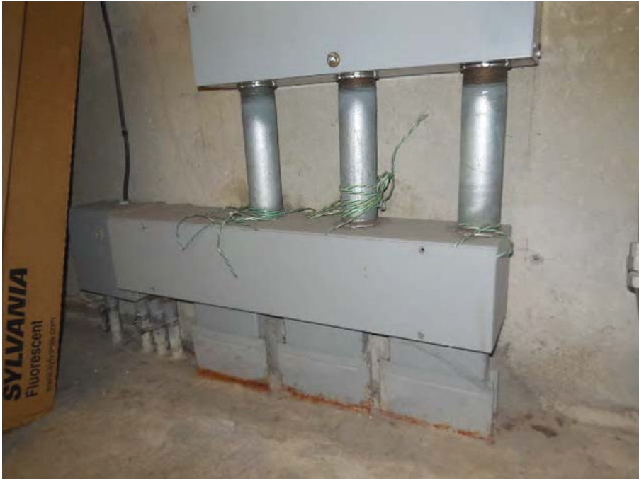
Photo #5: J03 Franconia-Springfield – Ducts feeding into trough in Room 216
