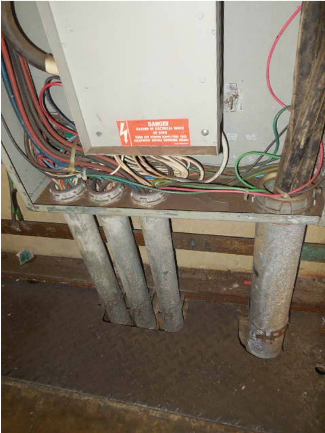
Picture 8: G02 Capitol Heights – AFC Panel MF in room 206 – Bottom conduits
