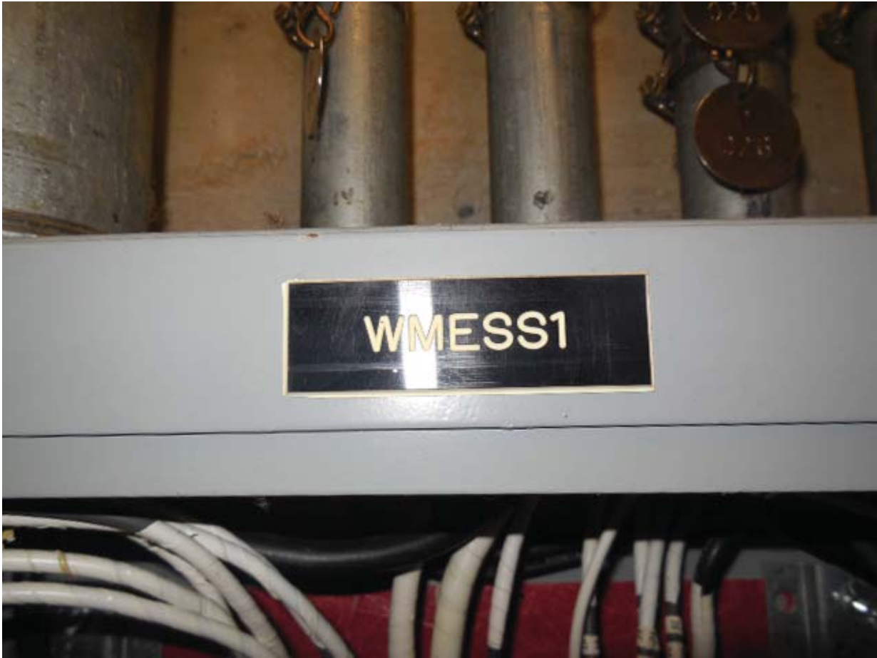
Picture 4: G05 Largo Town Center – AFC Panel WMESS1 in Room 117
