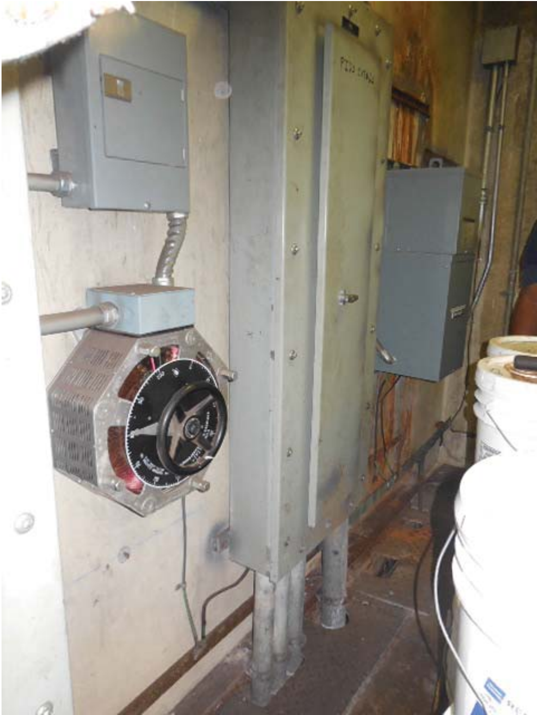
Picture 17: G02 Capitol Heights – Common trench in room 206
