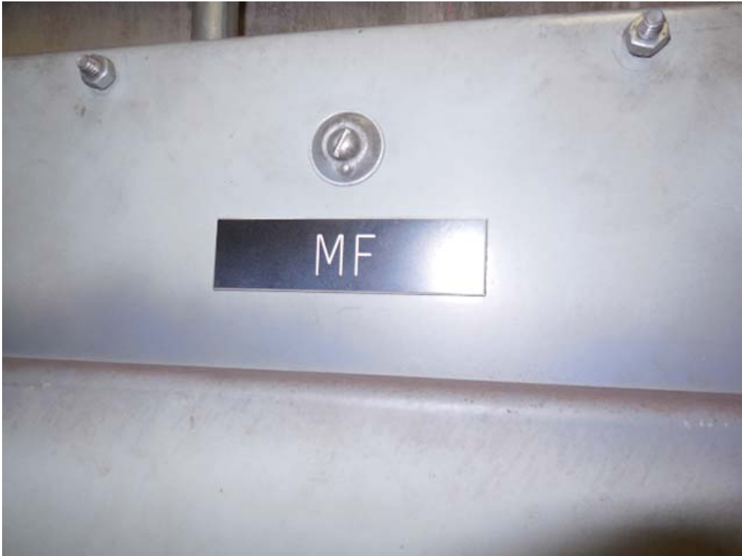
Picture 6: G02 Capitol Heights – AFC Panel MF in room 206
