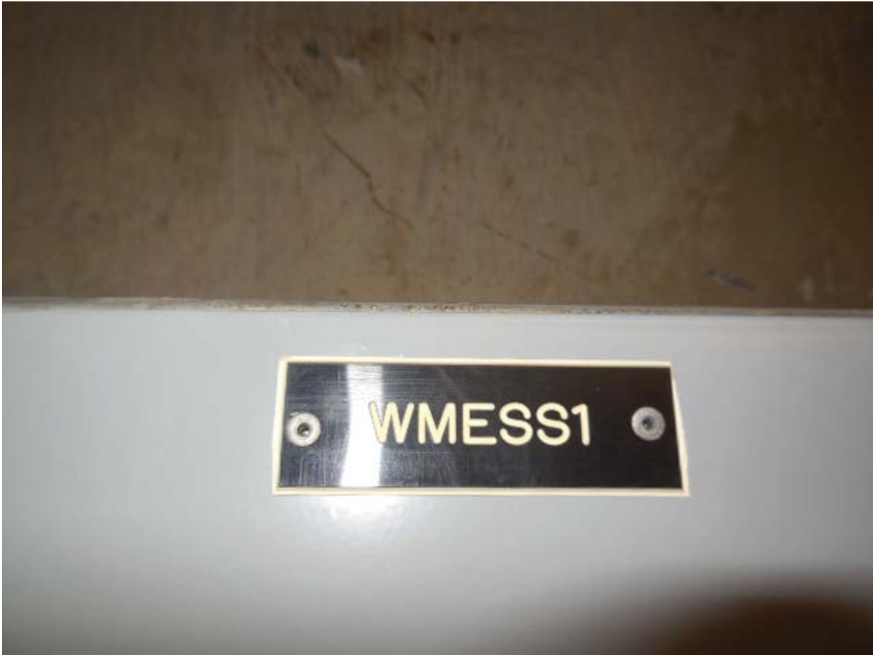
Picture 5: G04 Morgan Boulevard – AFC Panel WMESSI in Room 205
