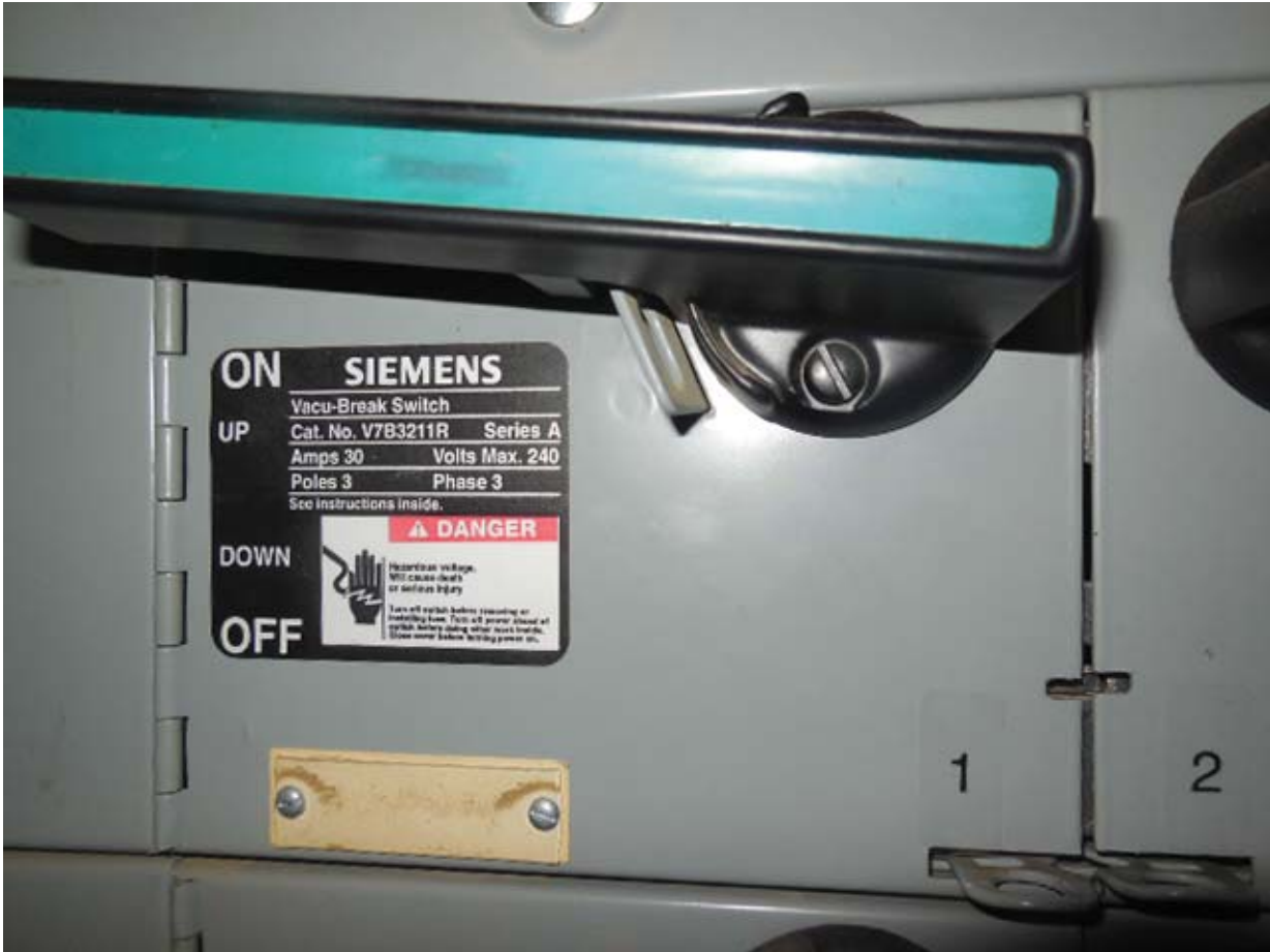
Picture 9: G05 Largo Town Center – Panel WMES Section 1 in Room 117 – Breaker 1
