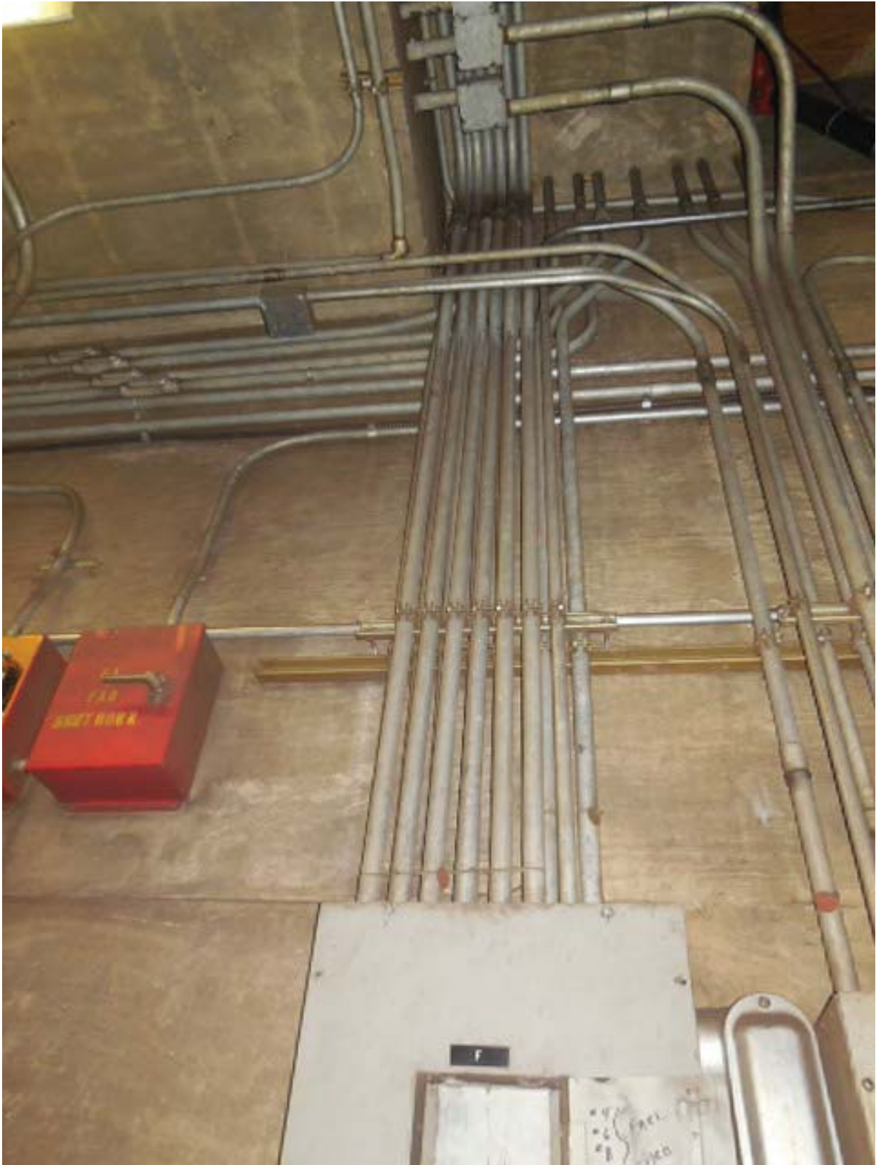
Picture 9: G01 Benning Road – AFC Panel F in Room 102 – Conduits above panel
