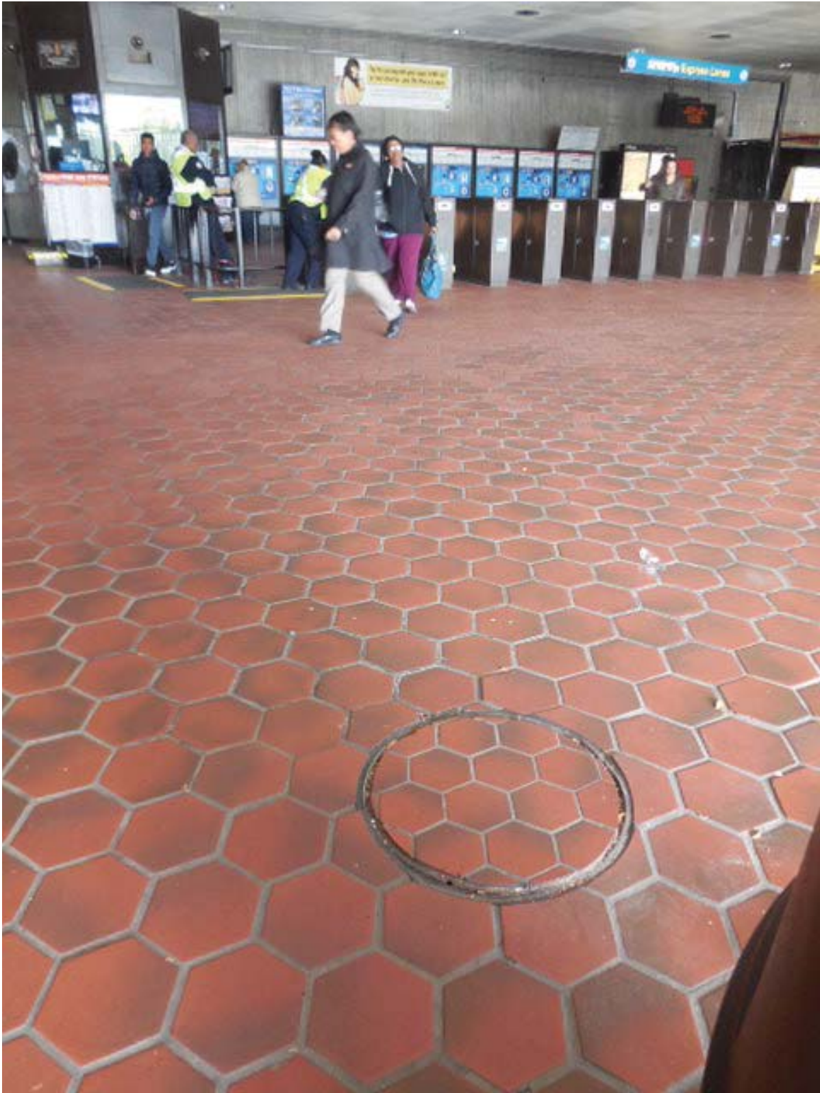
Picture 1: D13 New Carrollton – Handholes in Mezzanine
