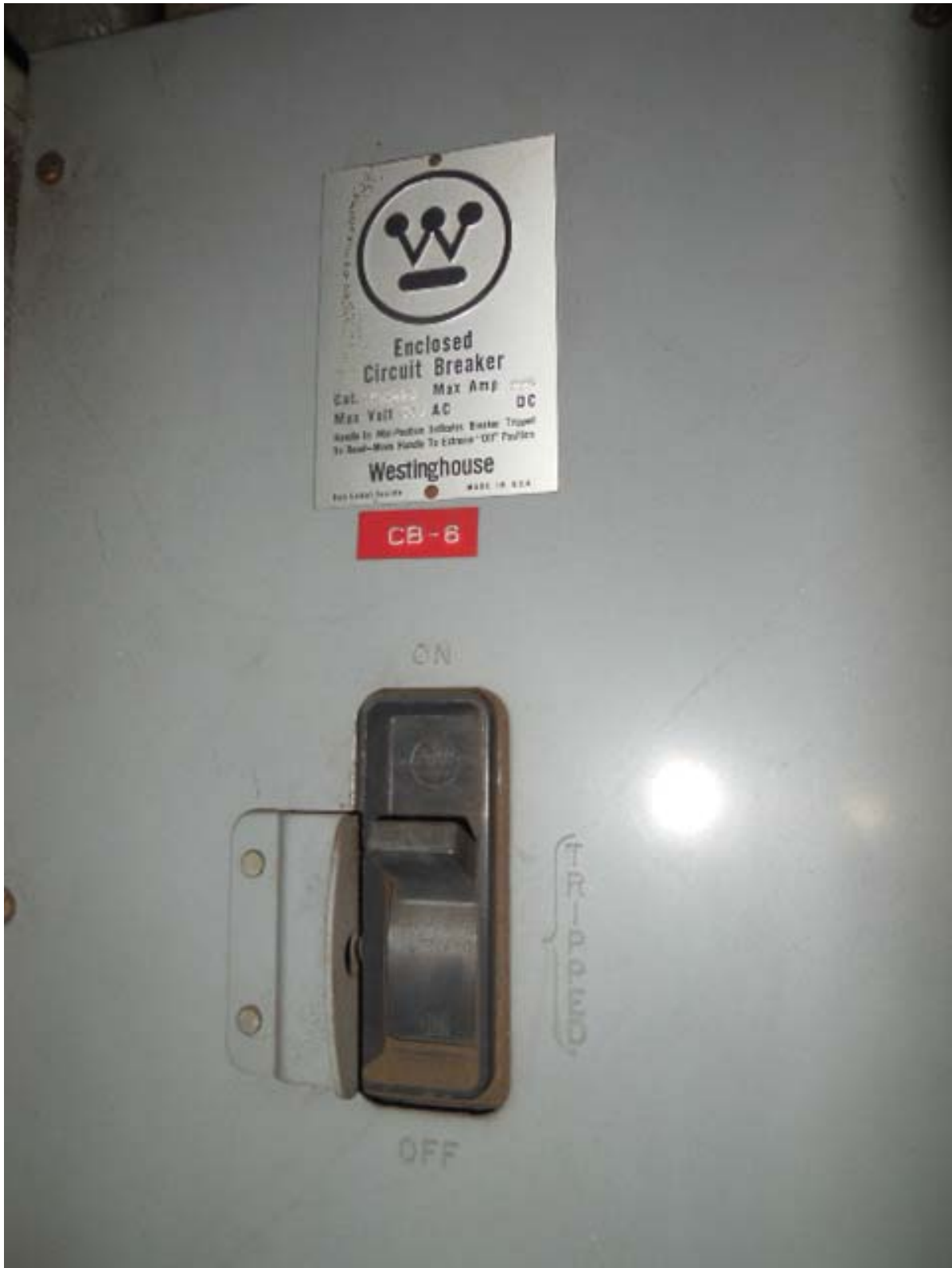
Picture 14: G03 Addison Road – DB-6 Disconnect switch in Room 207
