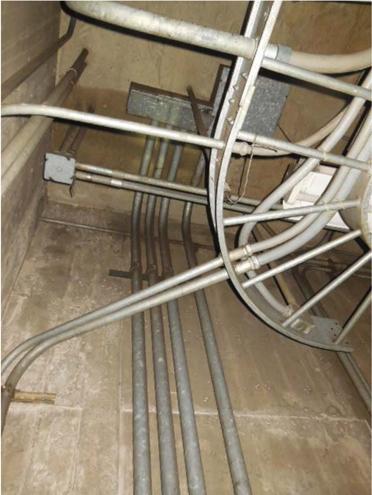
Picture 6: G03 Addison Road – AFC Panel F in Room 207 – Conduits above panel
