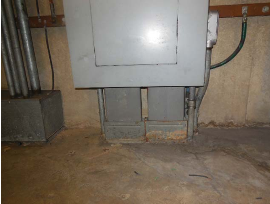
Photo #3: J02 Van Dorn Street – Ducts feeding into bottom of AFC panel NF in Room 110
