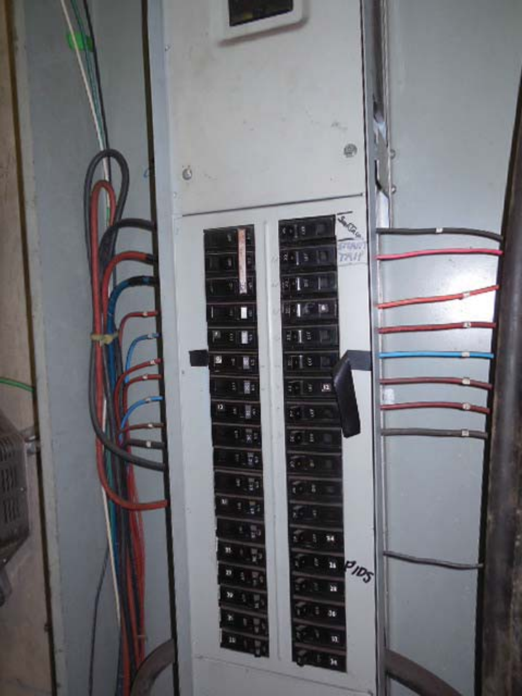
Picture 7: G02 Capitol Heights – AFC Panel MF in room 206
