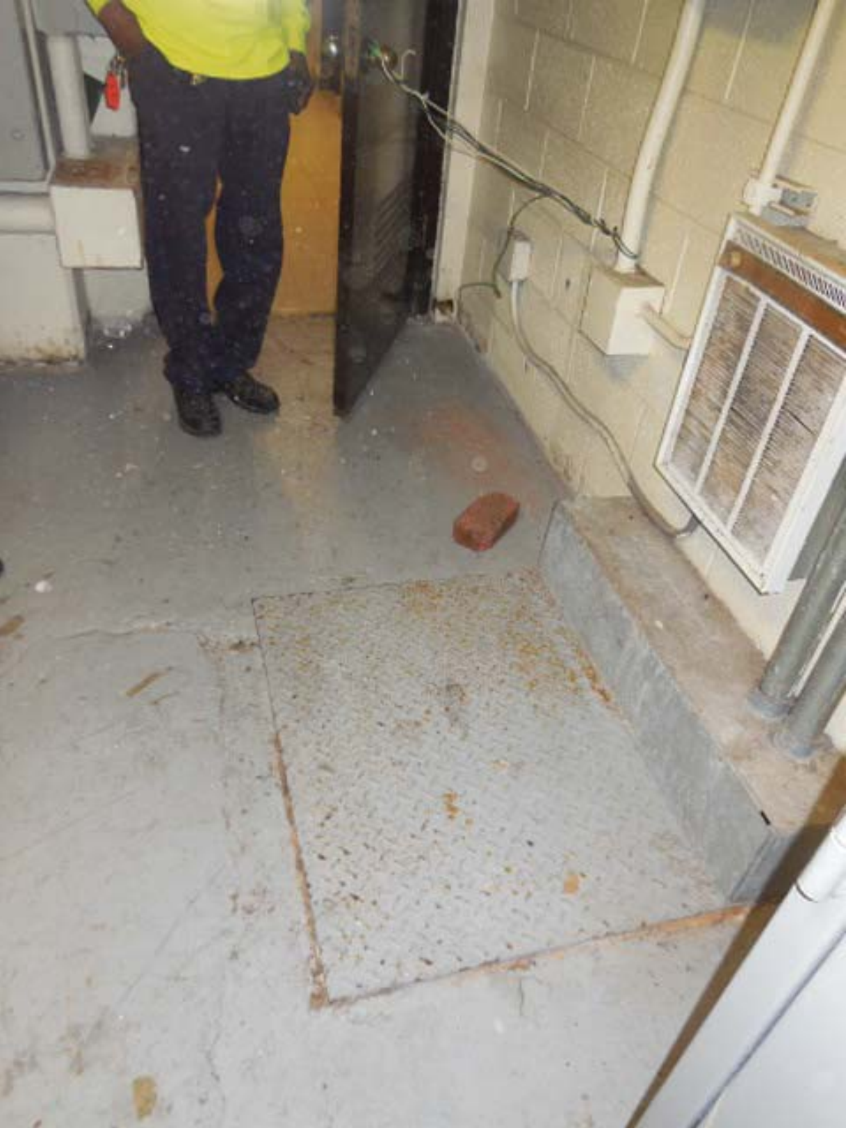
Picture 2: D13 New Carrollton – Steel plate on floor in Room C105
