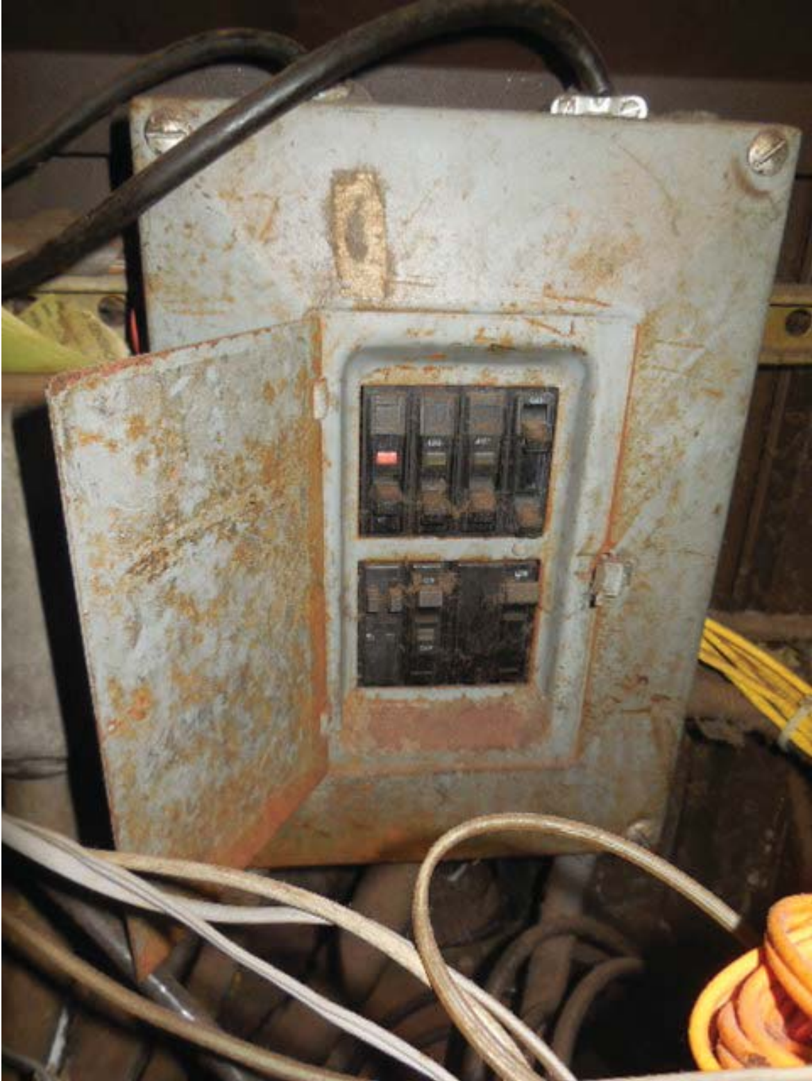
Picture 3: D13 New Carrollton – Emergency Panel in Kiosk
