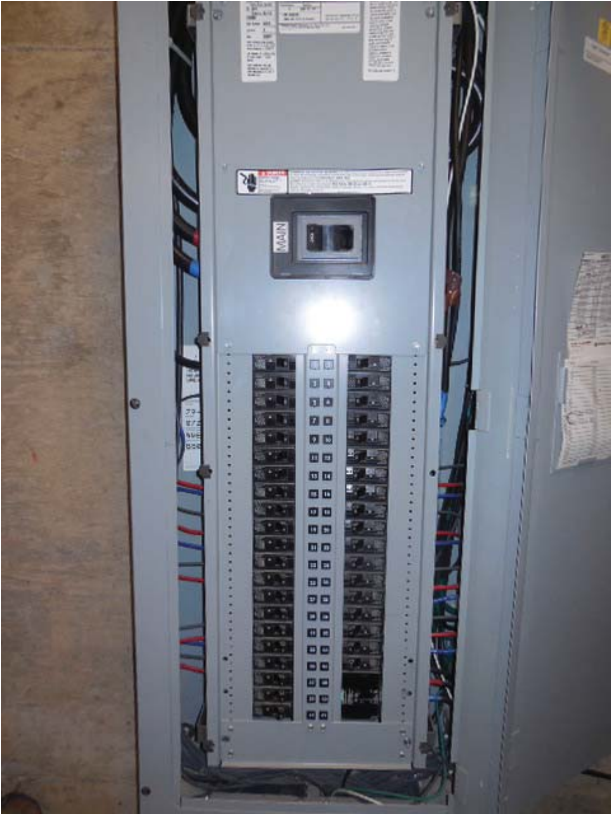
Picture 5: G05 Largo Town Center – AFC Panel WMESS1 in Room 117
