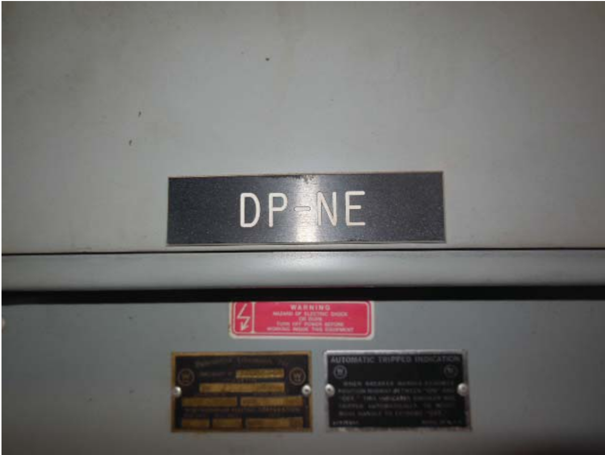
Picture 4: D13 New Carrollton – Source Panel DP-NE in Room 211
