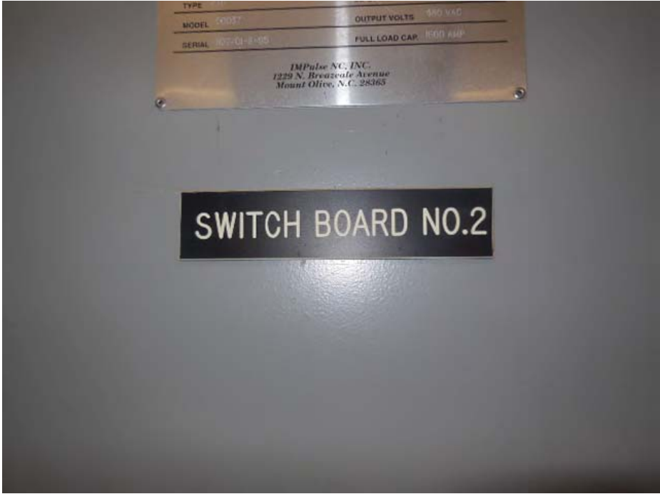
Photo #9: J03 Franconia-Springfield – Switchboard #2 label in room 216
