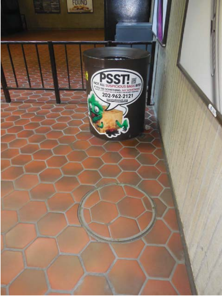
Photo #2: J02 Van Dorn Street – Mezzanine Level Handhole
