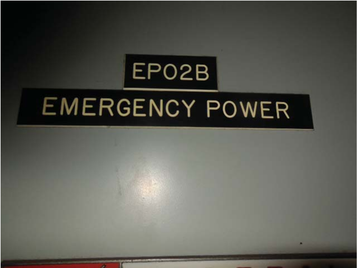
Picture 11: G03 Addison Road – EP02B Emergency Power Panel
