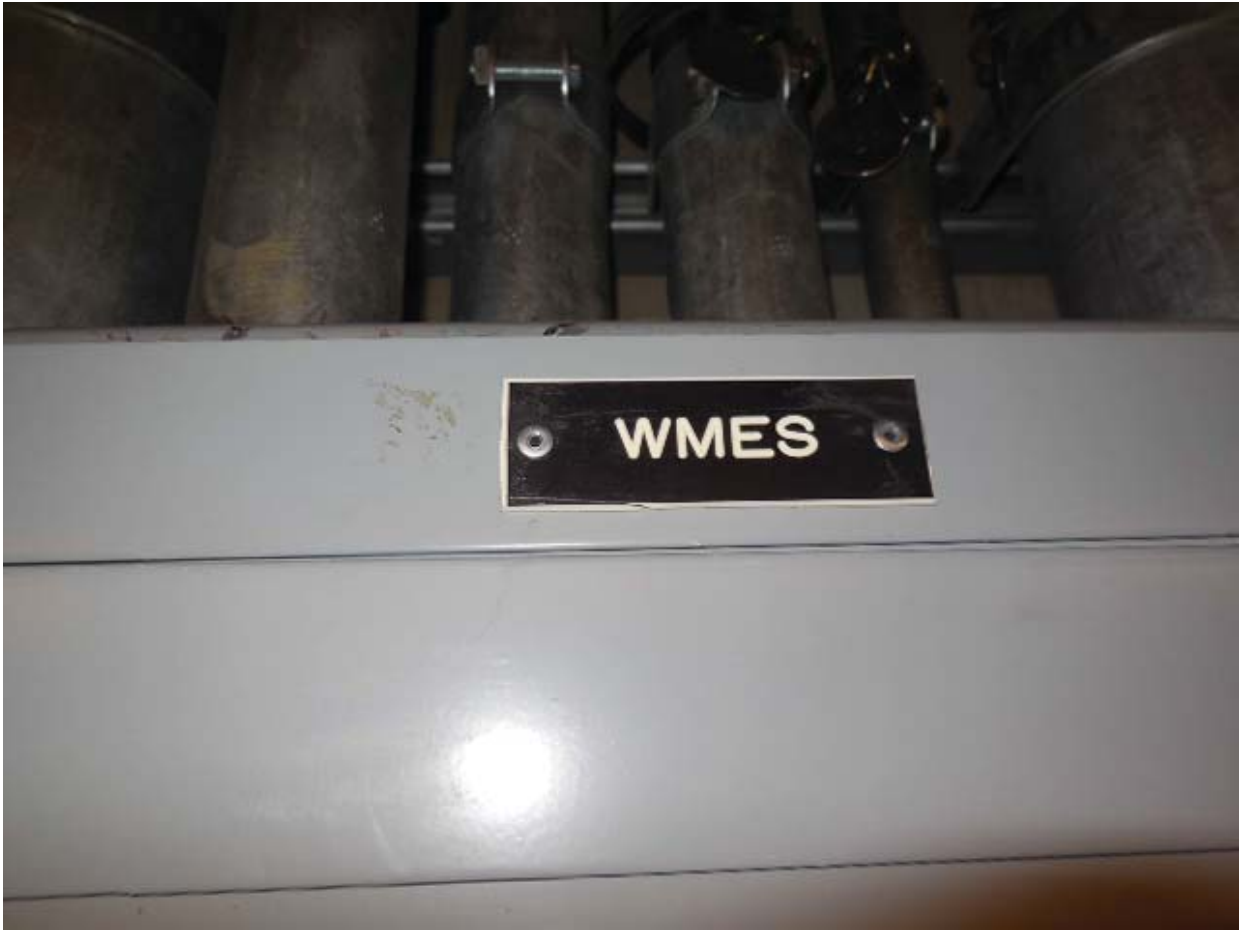
Picture 8: G04 Morgan Boulevard – Panel WMES in Room 205
