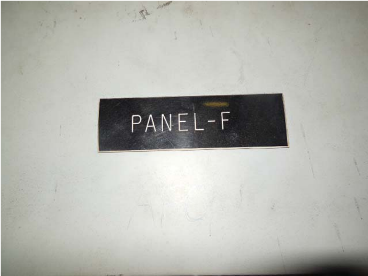
Picture 3: G03 Addison Road – AFC Panel F in Room 207
