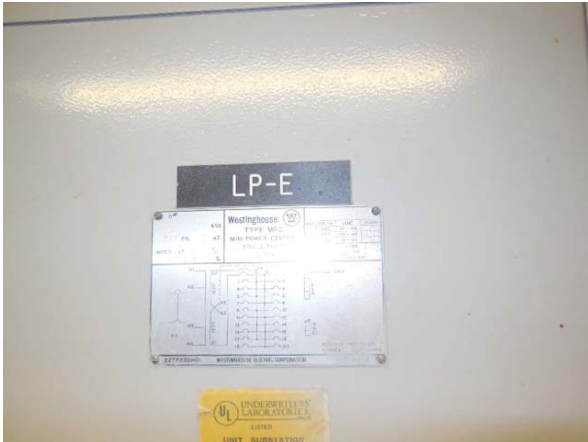
Picture 6: D13 New Carrollton – Panel LP-E in Room C106
