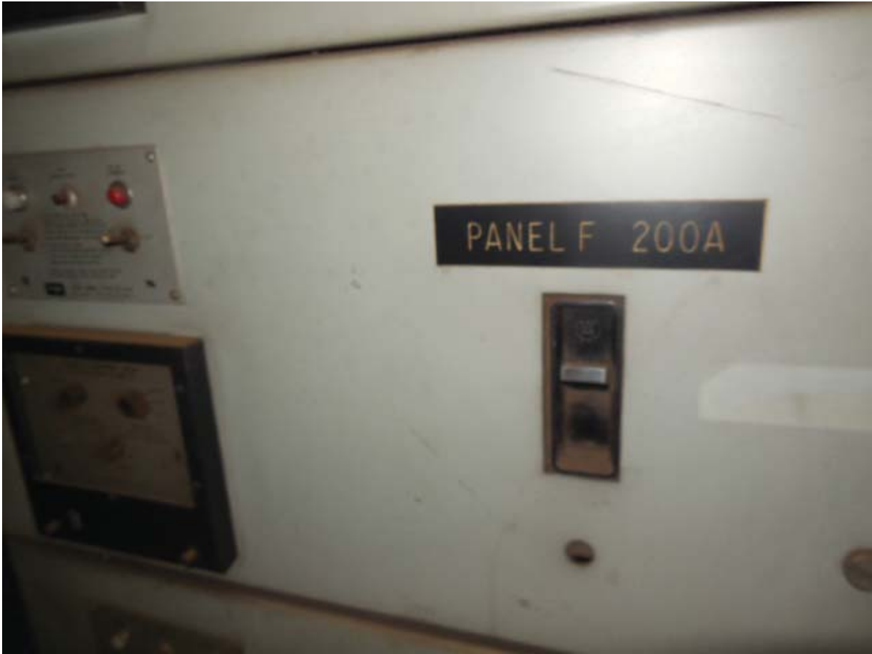
Picture 12: G01 Benning Road – West AC Substation Switchboard in Room 203 – Circuit 9 for AFC Panel F
