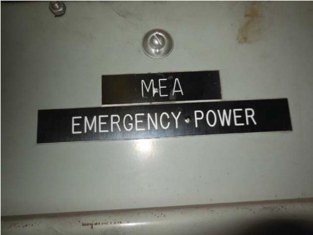
Picture 9: G02 Capitol Heights – Emergency power Panel MEA in room 206
