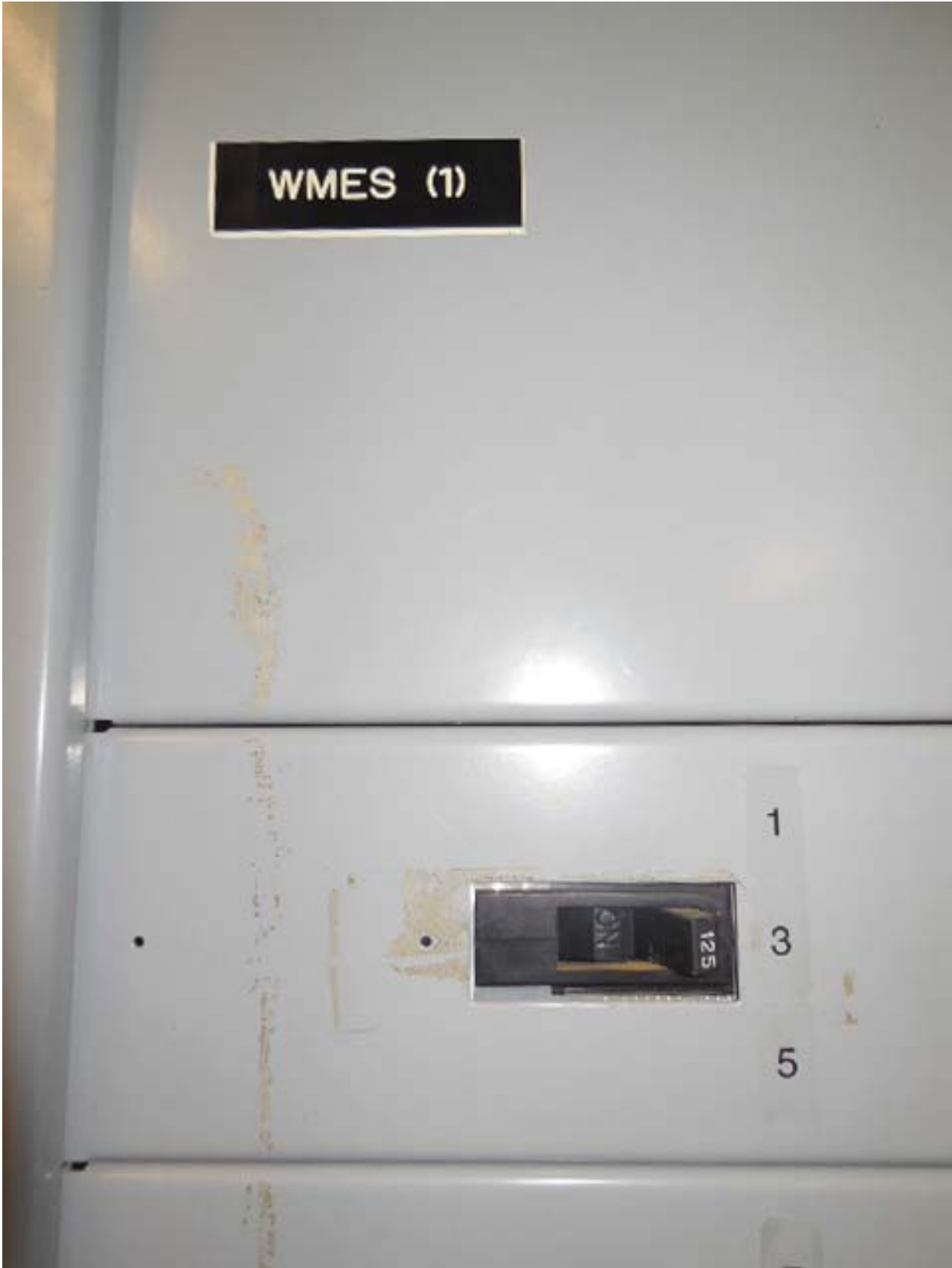
Picture 8: G05 Largo Town Center – Panel WMES Section 1 in Room 117
