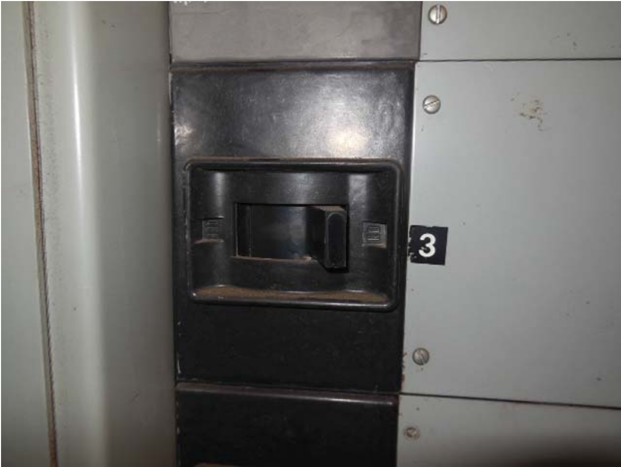
Picture 5: D13 New Carrollton – Source Panel DP-NE Breaker #3 in Room 211
