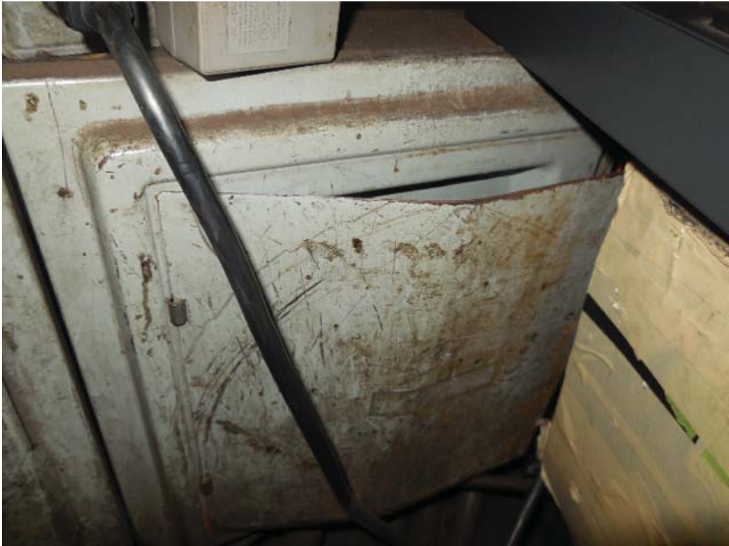
Pictures 4&5: G02 Capitol Heights – Emergency panel in Kiosk
