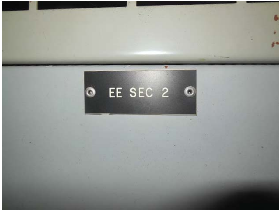
Photo #11: J03 Franconia-Springfield – Emergency feed for Kiosk Panel – Source Panel EE Label
