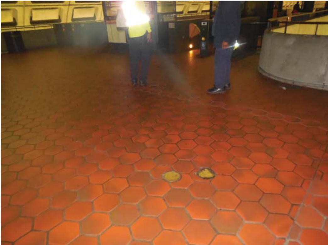
Pictures 1&2: G02 Capitol Heights – Handholes in mezzanine
