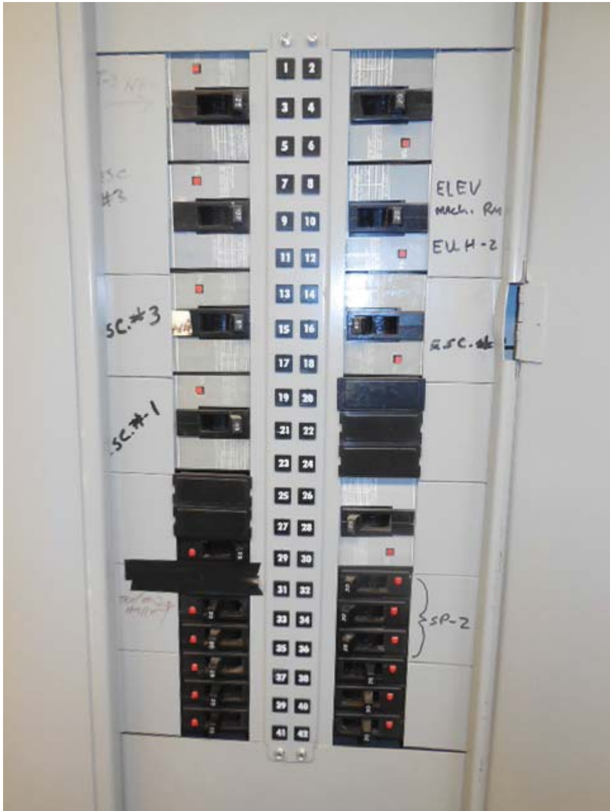
Picture 9: G04 Morgan Boulevard – Panel WMES in Room 205
