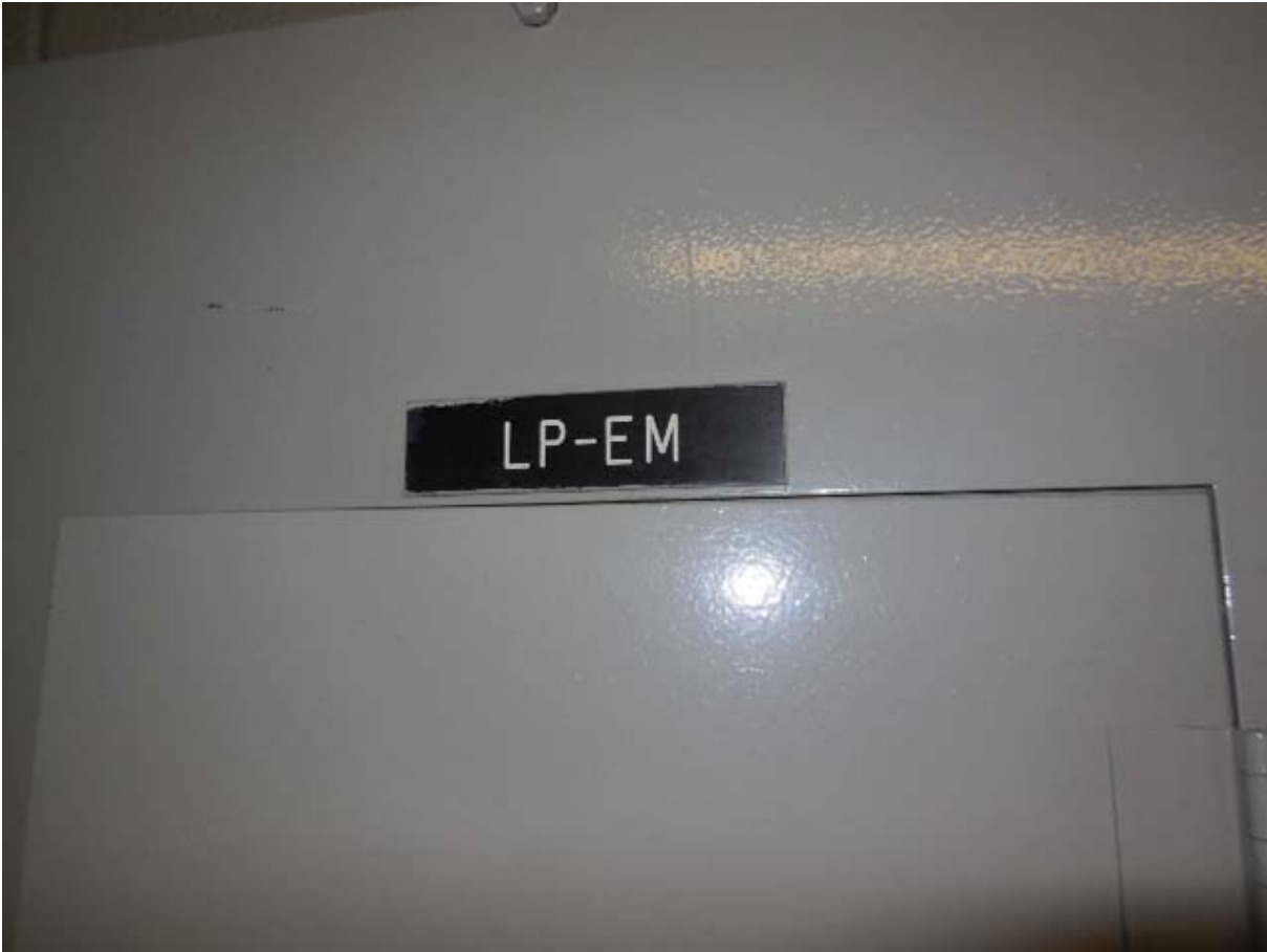
Picture 7: D13 New Carrollton – Panel LP-EM in Room C106
