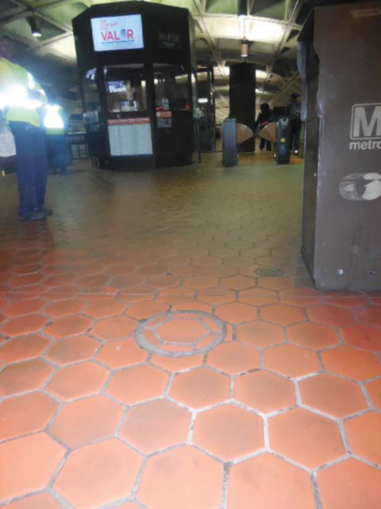
Picture 1: G01 Benning Road – Manhole & handhole in Mezzanine
