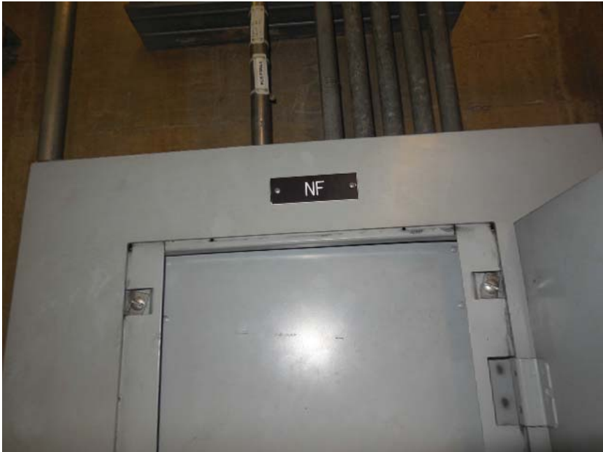
Photo #6: J02 Van Dorn Street – Label of AFC panel NF in Room 110
