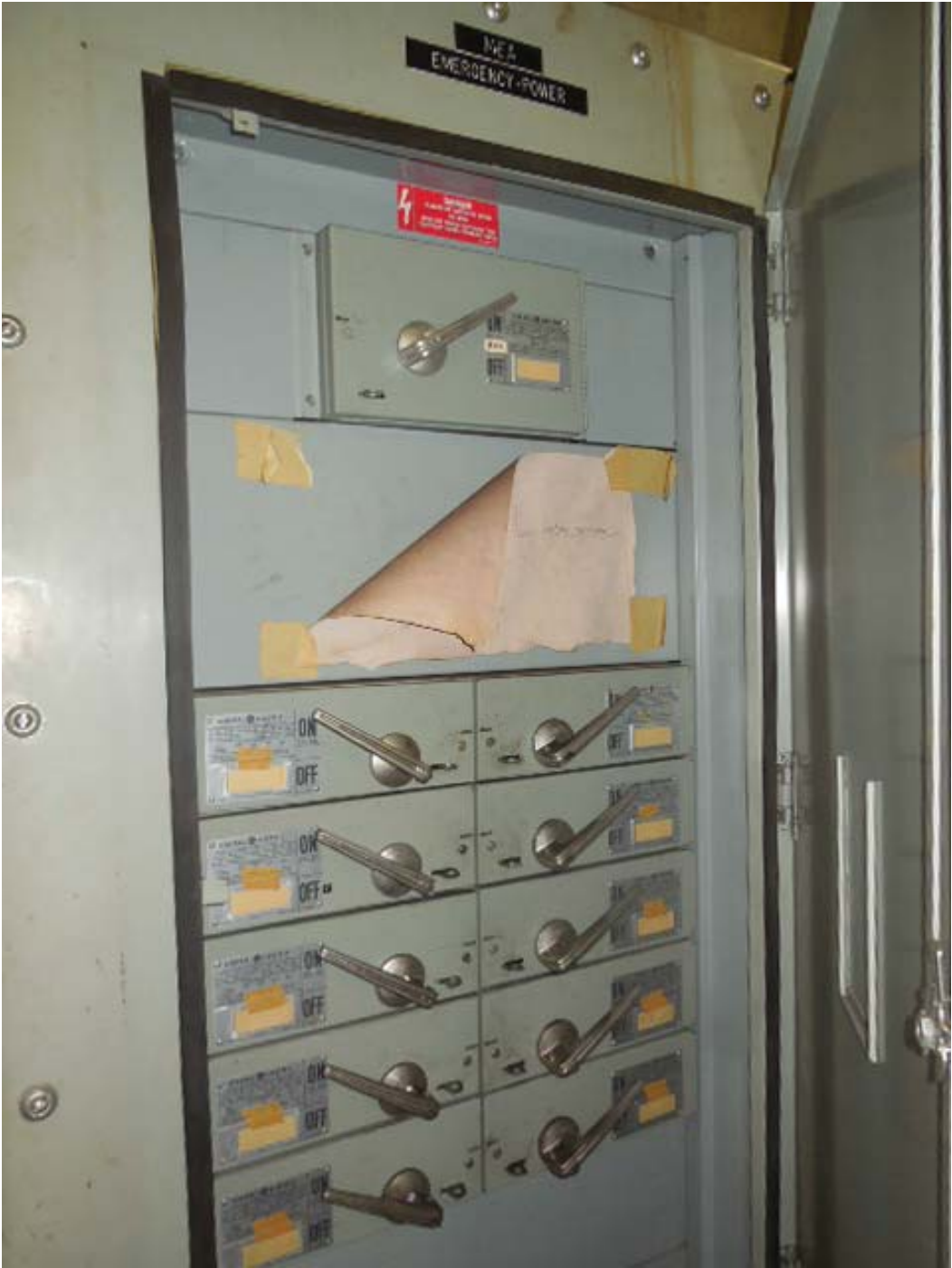
Picture 10: G02 Capitol Heights – Emergency power Panel MEA in room 206
