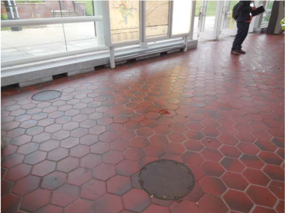
Picture 2: G04 Morgan Boulevard – Manholes in Mezzanine
