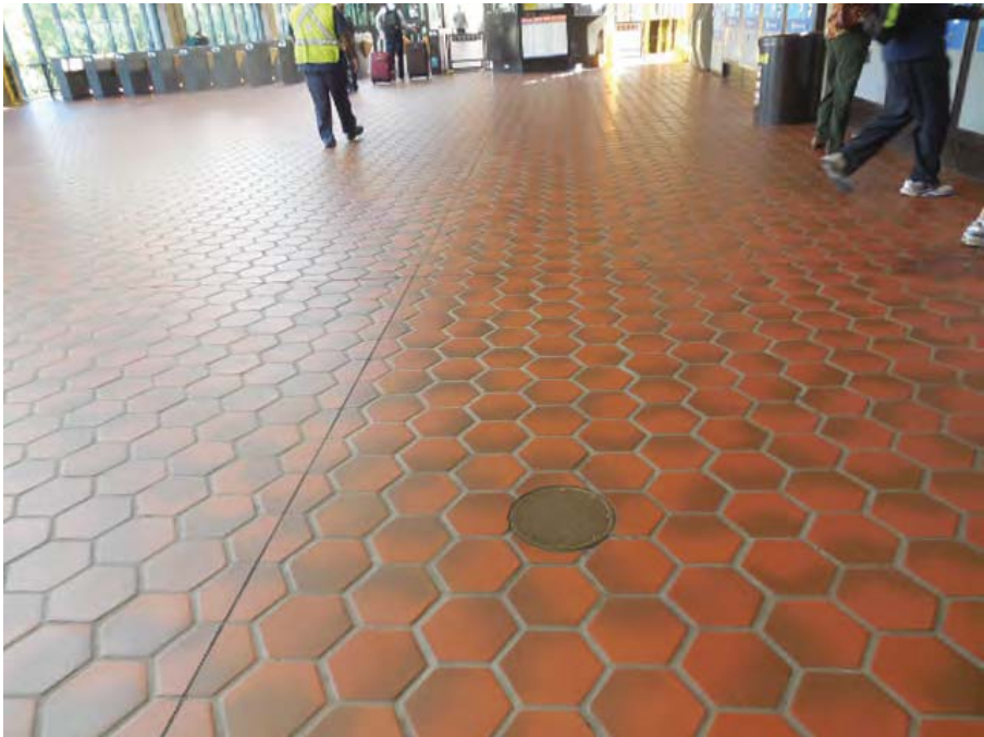
Photo #4: J03 Franconia-Springfield – Handholes in mezzanine floor
